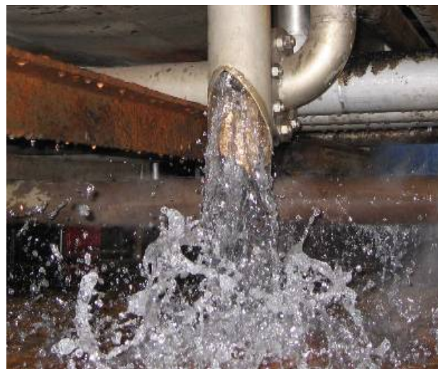
Plate 1.1. Water losses from the pasteuriser pipe A
