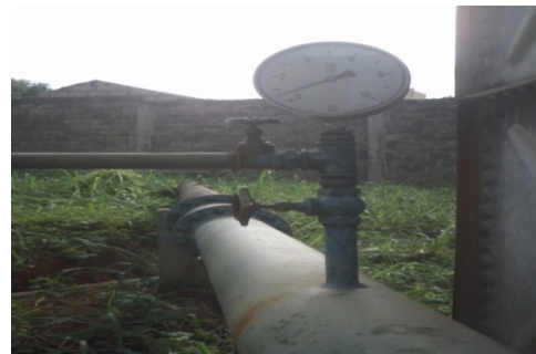
Plate 4.1. Gauge Meter for the Water Treatment Plant
